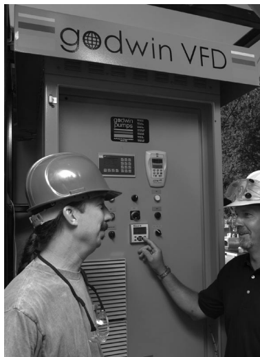
The pumps were controlled by VFDs incorporating level transducers and PLCs.
